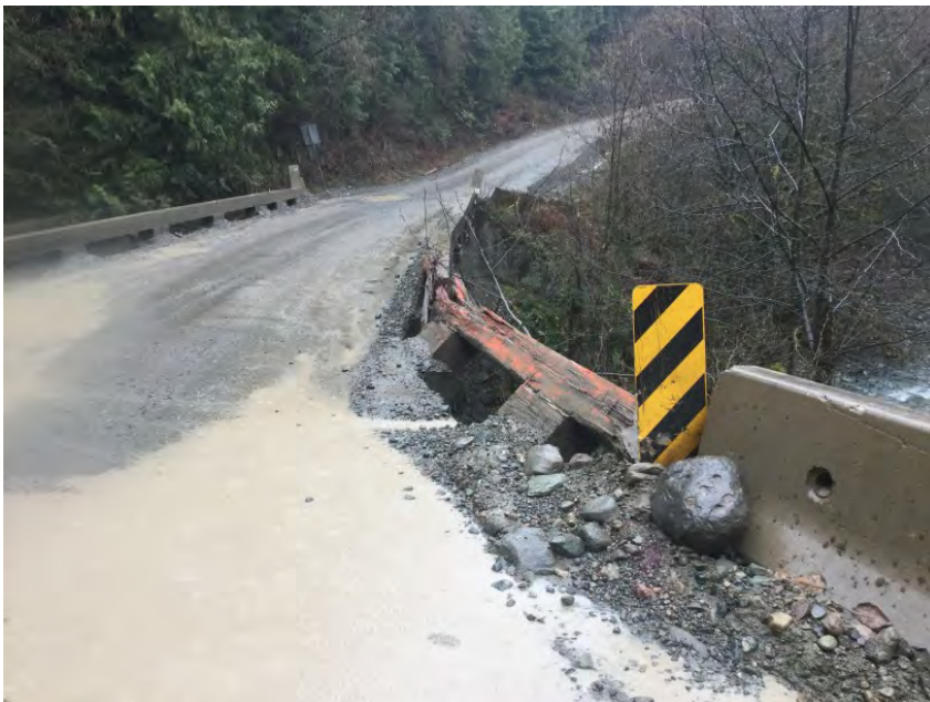
Dam aged guardrail
